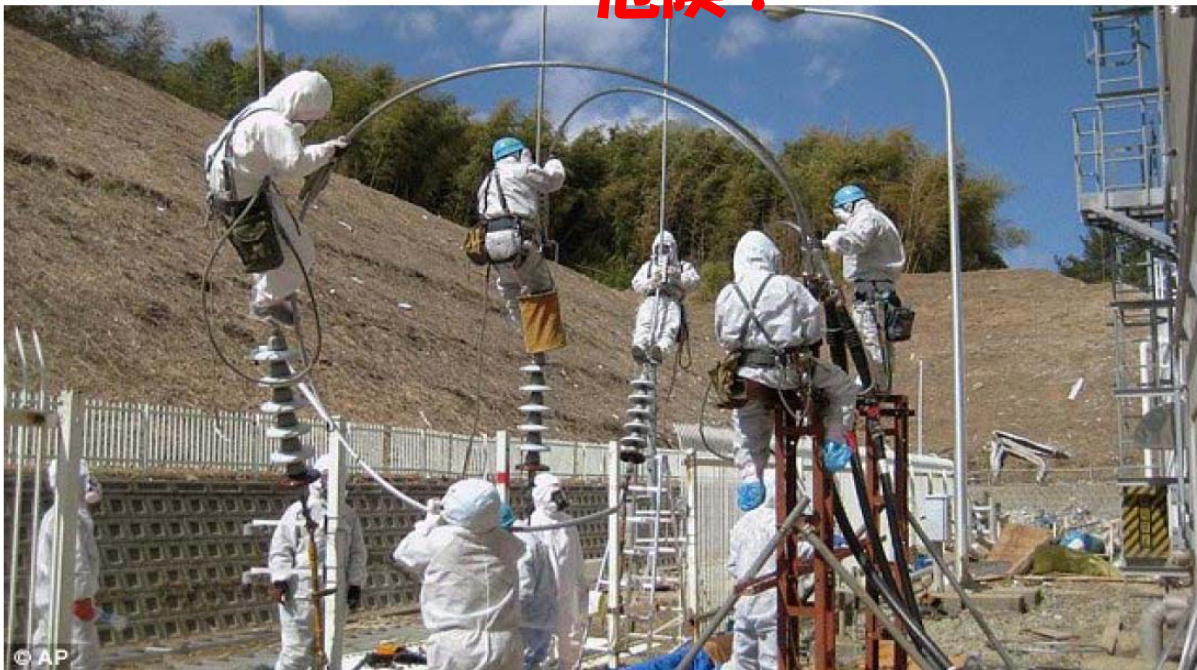
Teamwork: Outside the men connect transmission lines to restore electric power supply to Unit 3 and Unit 4
